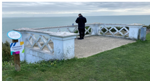
Leas Balcony, Clifton Crescent before repainting.
